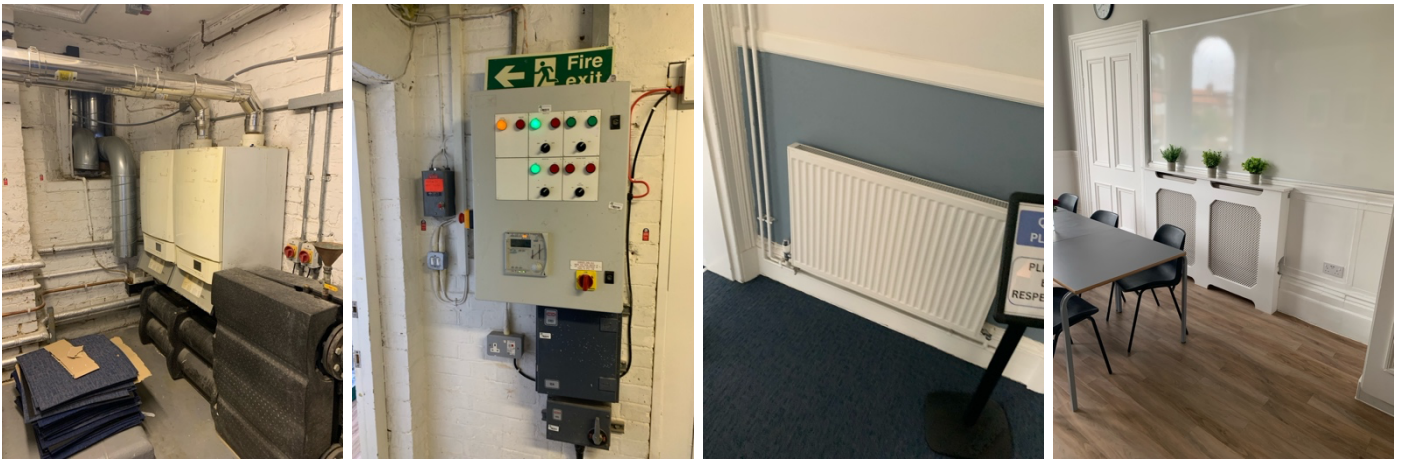
Figure 2: (A) and (B) Heating system. (D) and (C) Examples of the radiators throughout the building.
